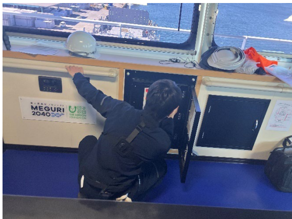
Checking the fire control panel
