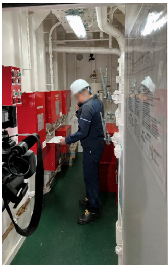
Communication with the fire control room
